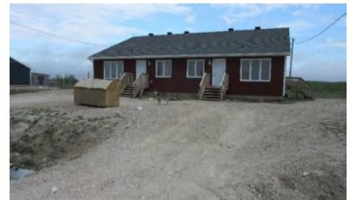
Sloping the ground around houses helps water drains away from the foundation into the ditch.
