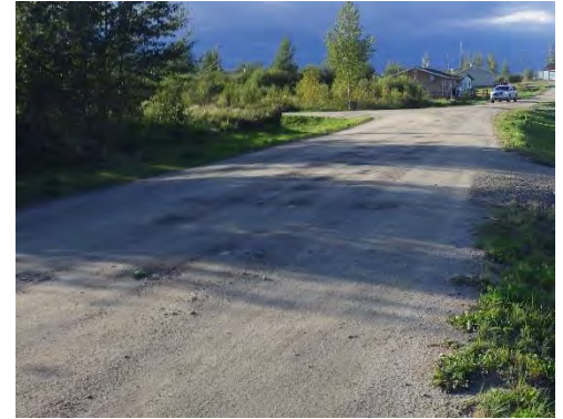
Dirt and gravel roads can become marked with potholes when water doesn't drain away properly.
