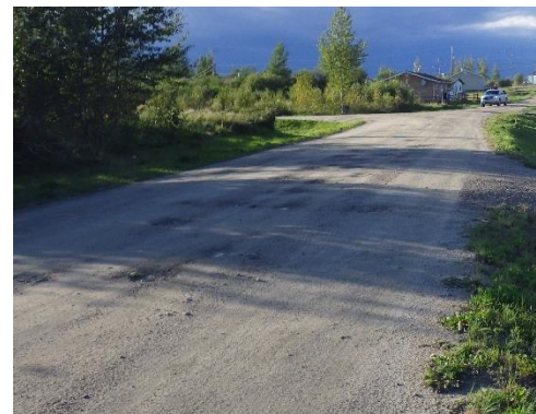
Dirt and gravel roads can become marked with potholes when water doesn't drain away properly.
