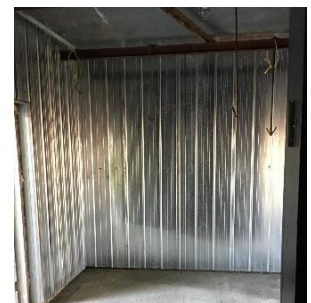
Inside of community cooler in Chapleau Cree First Nation Photos by Dakota Souliere.
