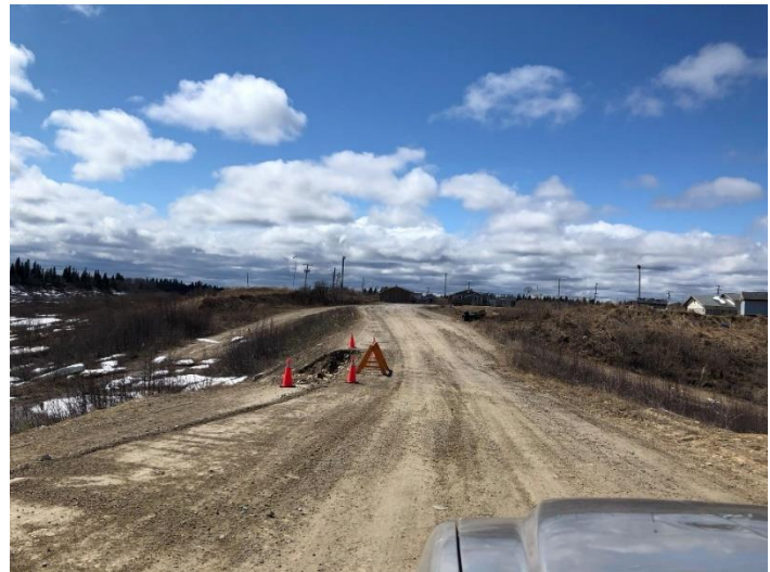
ROAD WASHOUT, ANDERSON DYKE, FORT ALBANY, PHOTO FROM FORT ALBANY FLOOD WATCH FACEBOOK PAGE
