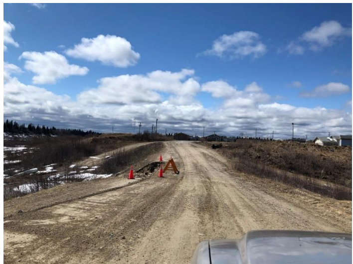
ROAD WASHOUT, ANDERSON DYKE, FORT ALBANY, PHOTO FROM FORT ALBANY FLOOD WATCH FACEBOOK PAGE
